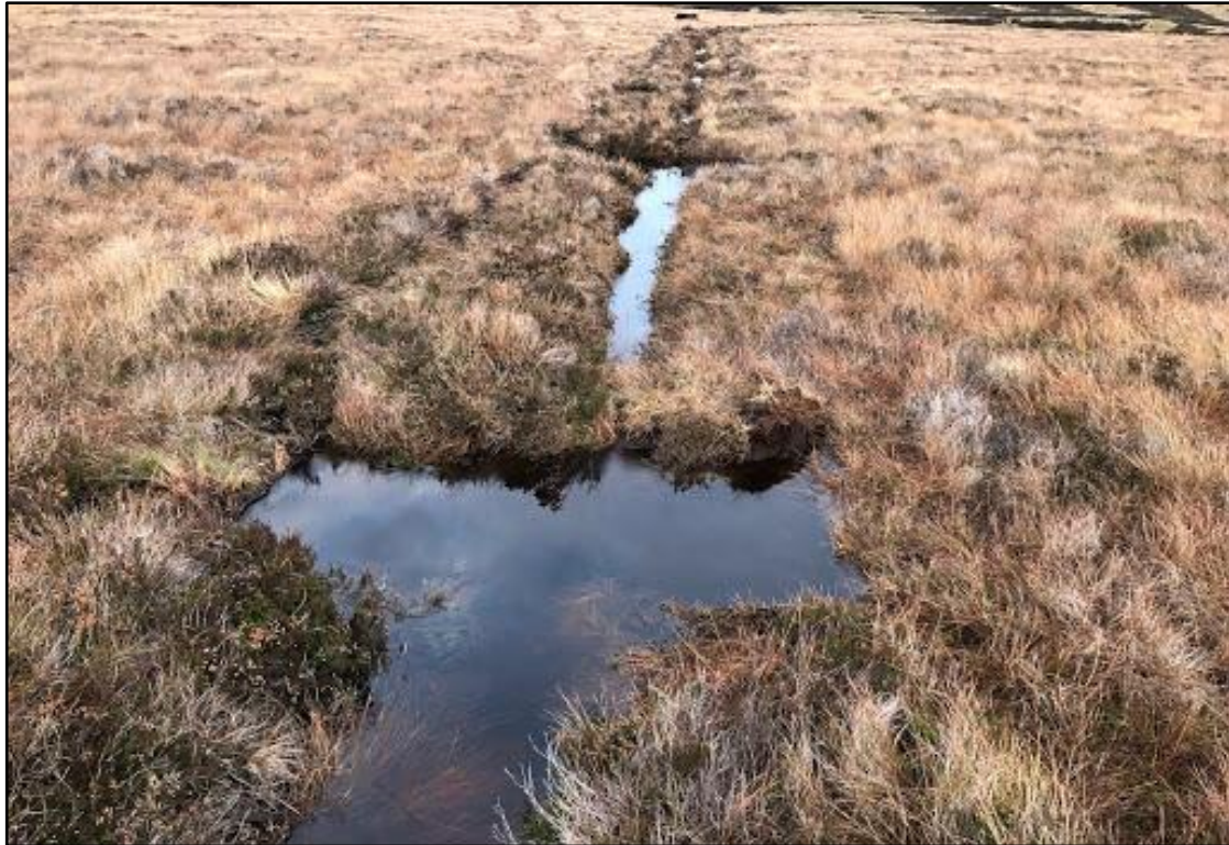
Plate 2-2. Example of peat dams to be used for on-site forestry drain blocking. This will re-establish and maintain a hydrological regime for the required peatland rehabilitation.
